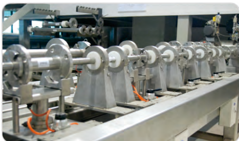
Piping system I (Max capacity for four meters calibration simultaneously in above system.)
