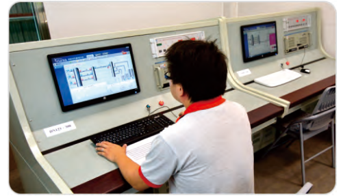
Control room & Graphical HMI
